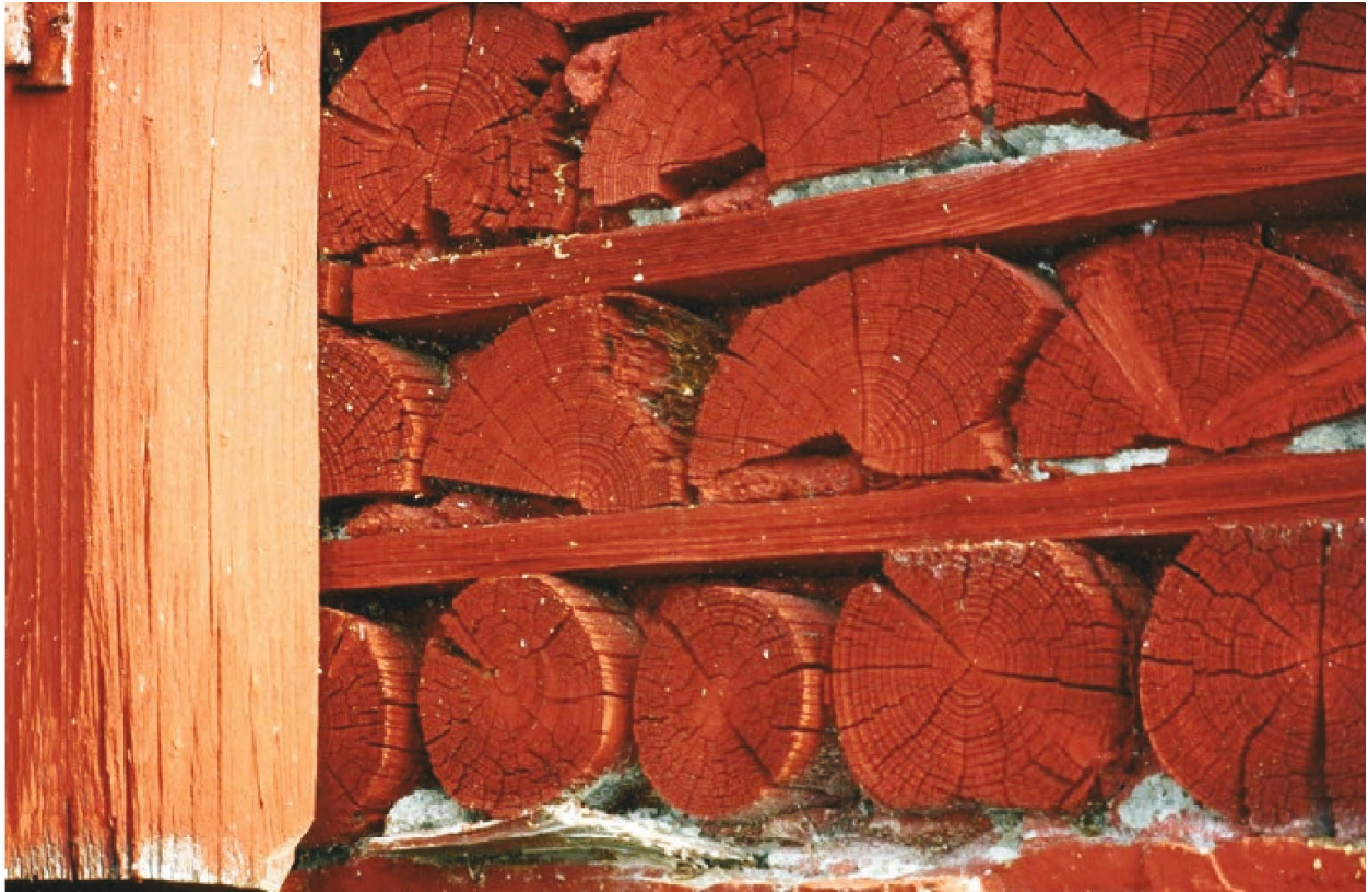
Fig. 23. A closeup of the wall seen in Fig. 22. There is for the most part wood resting on wood, so there is continuous vertical wood on wood contact. In this case the wood can be said to be load bearing for the most part alone [SINTEF Byggforsk, 2017, p. 3].
